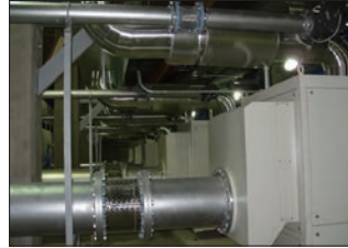
Suji WWTP (NX300), Korea
